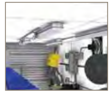
Full Electrical Service
